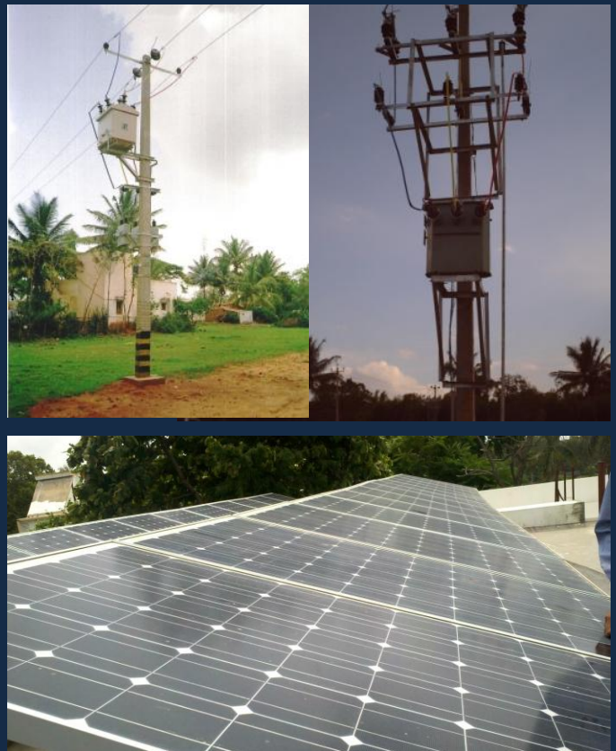
Above: Projects supported by DRUM: the Distribution Reform, Upgrades and Management Program. (Top two photos courtesy of USAID/India; bottom photo by Melissa Fraser, USDA)
